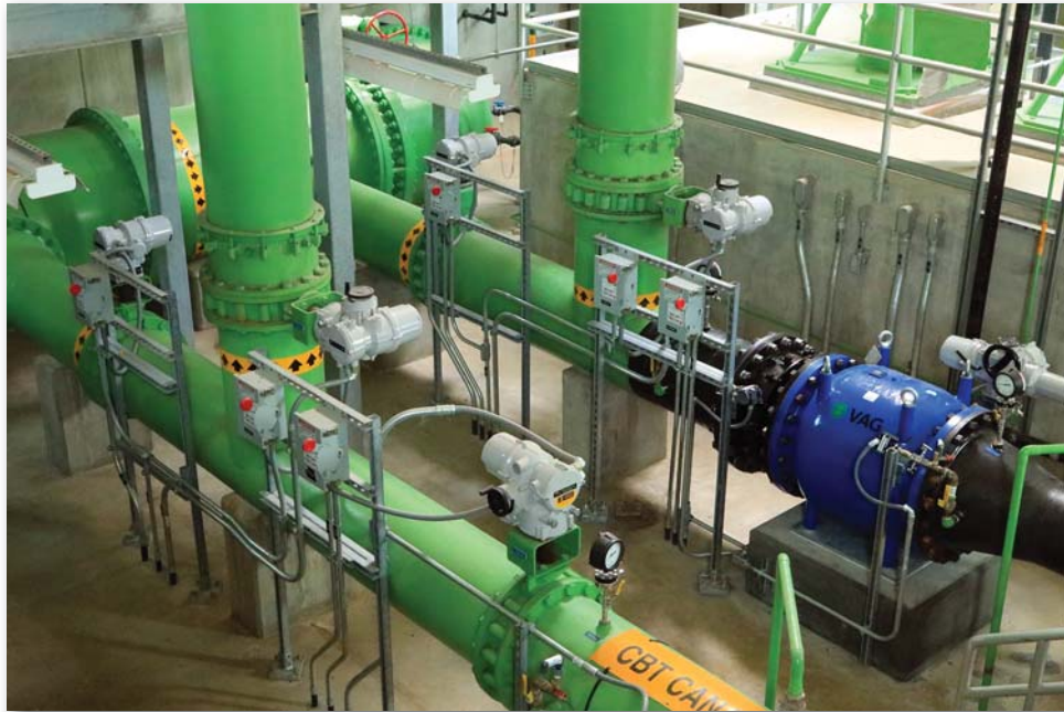
The City of Longmont's blending structure, where four different raw water sources are received, metered and blended, then delivered to the forebay pond of the Nelson-Flanders water treatment plant.
